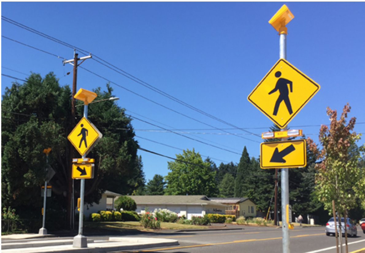
Figure 4: Rectangular Rapid Flashing Beacon
